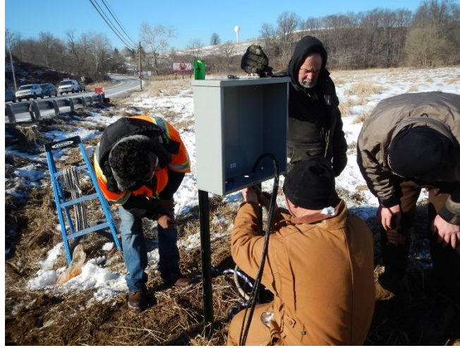
Figure 47. Electrical box for storing DAQ and electrical components for the second installation
