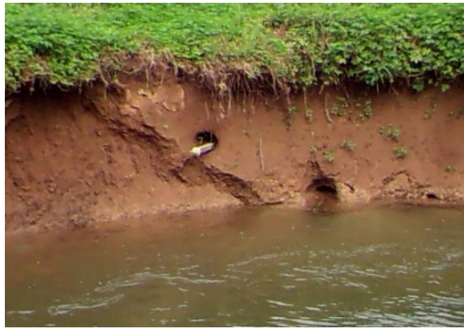
Figure 48. Residual cove formed from drilling
