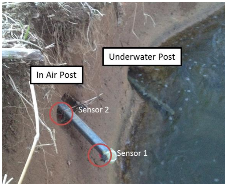
Figure 49. State of the lateral riverbed migration scour posts upon taking of data
